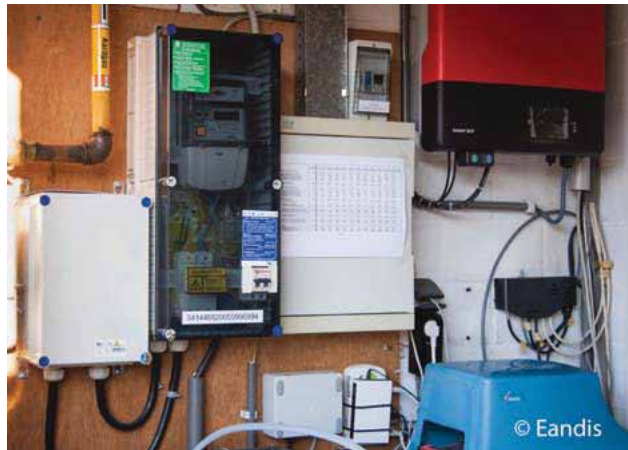
Figure 26: Linear installation including an Eandis smart meter
